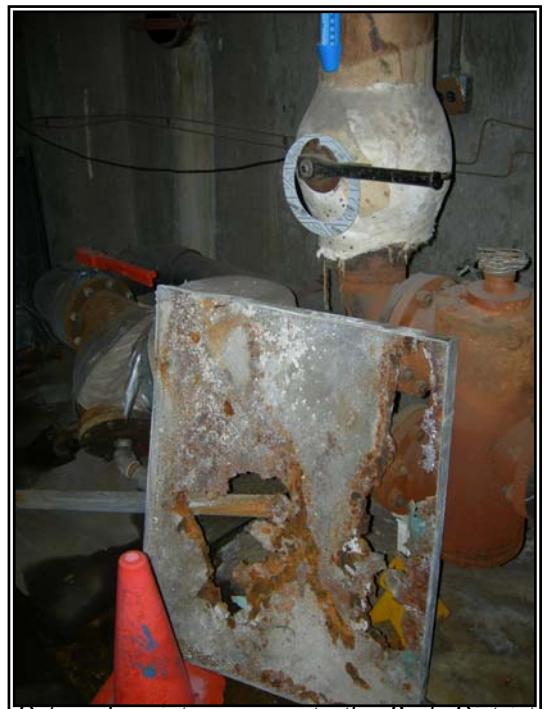
Deferred maintenance costs the Park District thousands of dollars each year and is the source of many system failures. These system failures are beginning to affect the Park District's programming on an increasing basis.
