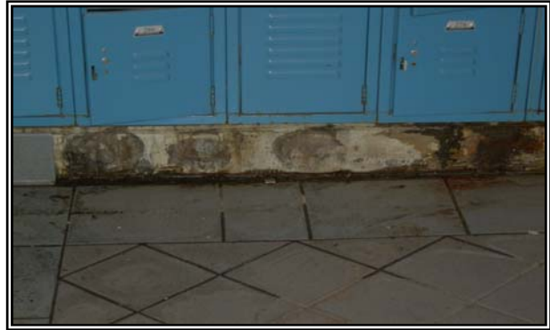
Despite recent renovations, many common areas at Ridgeland Common are in need of repair or replacement.
